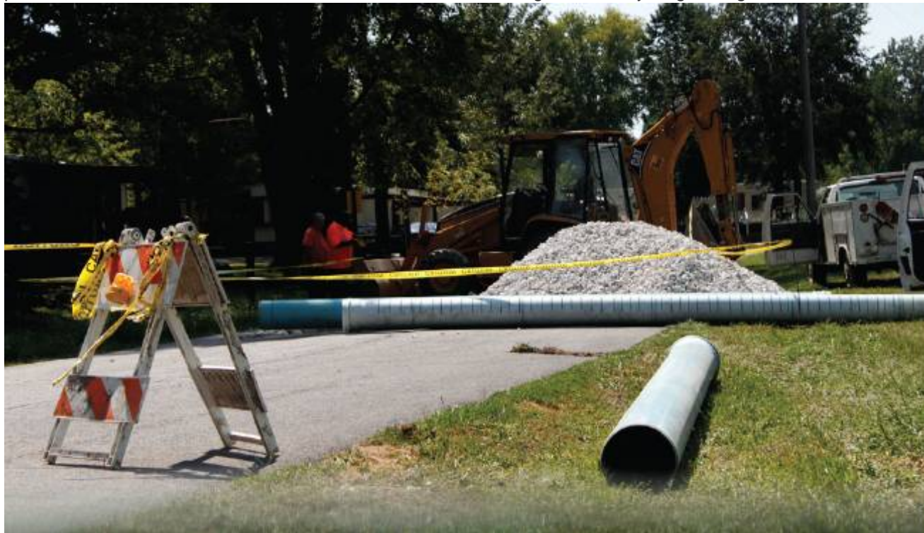
Alliance Water Resource employees work on sewer lines at Page Branch Park over the summer. This is just one of the projects done by Alliance.
